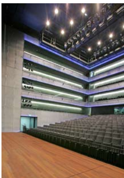
Loudspeakers for the MCR system are concealed behind the balconies' metallic fronts
