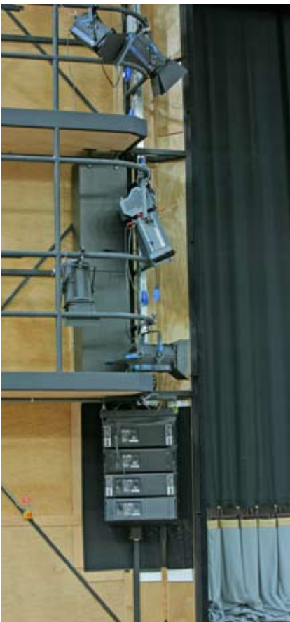
View from behind the proscenium arch, showing one of the XLNT Bassbeam subwoofers and a Martin line array cluster
